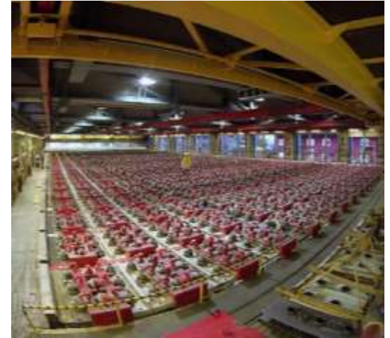
BASF 2010 View of a mercury cell room
